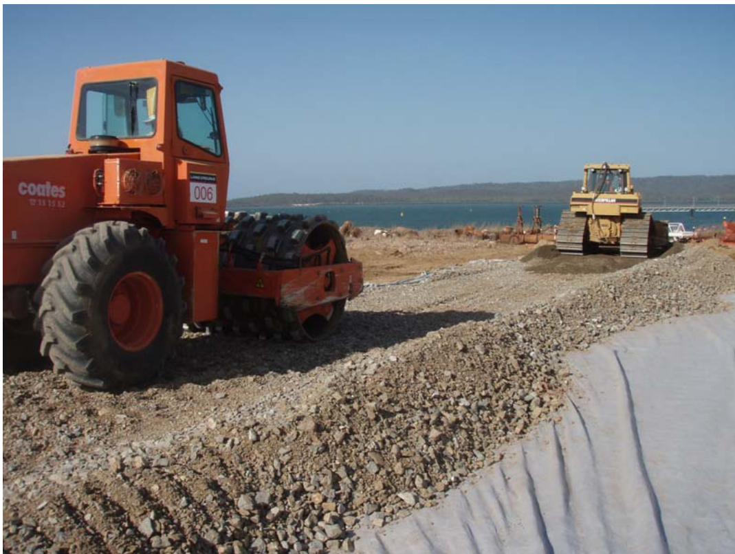
Preparation of cutter soil mixing (CSM) piling platform for trials that have now commenced on the LNG tank location.
