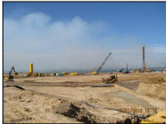
Figure 2: Formation of the haul road around the tank foundation visible in the foreground. Smoke from the burn-off on Curtis Island visible in the background.
